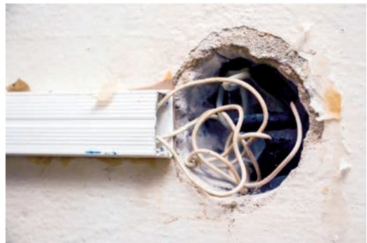
Fig. 1.28: Be careful of exposed cables
